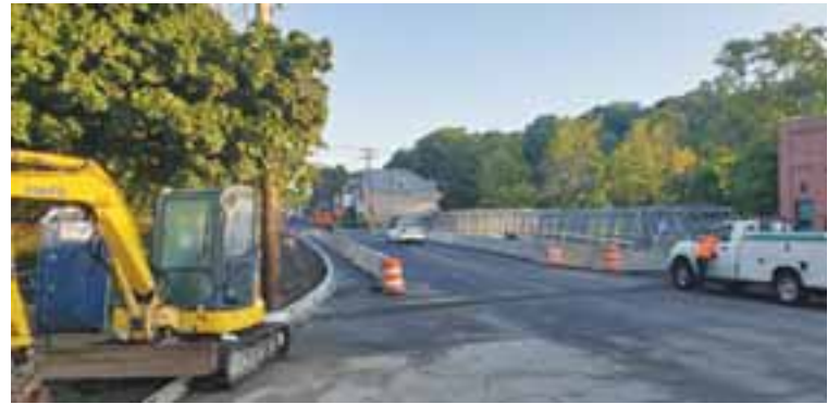
Work is still ongoing, but the bridge itself is ready to handle whatever traffic you can throw at it.
