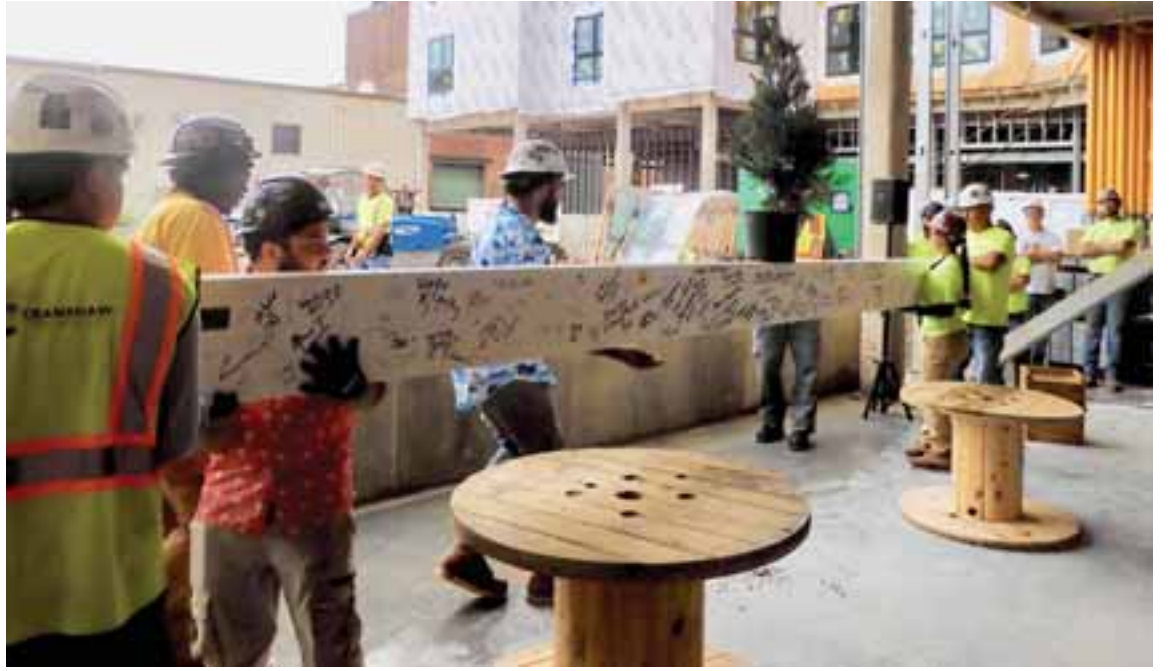
Workers carry the roof beam to the crane so it can be lifted to its final resting place.
