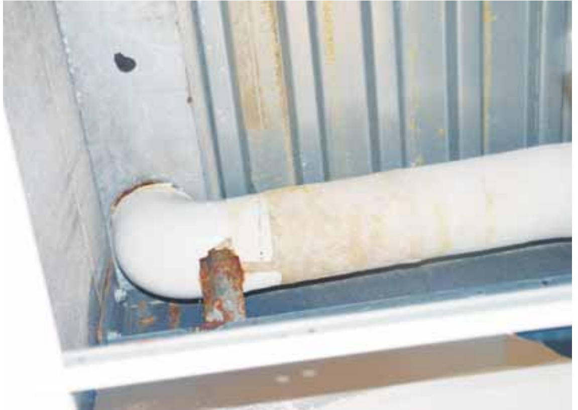
According to officials, the flooding appears to be coming from this pipe.
