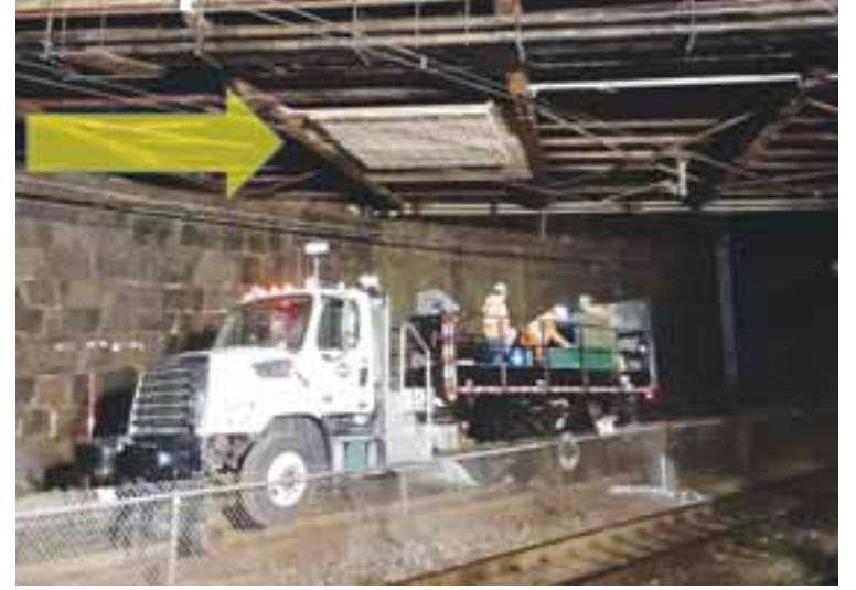
Work is progressing on the bridge project, if a bit slower than residents would probably like.
