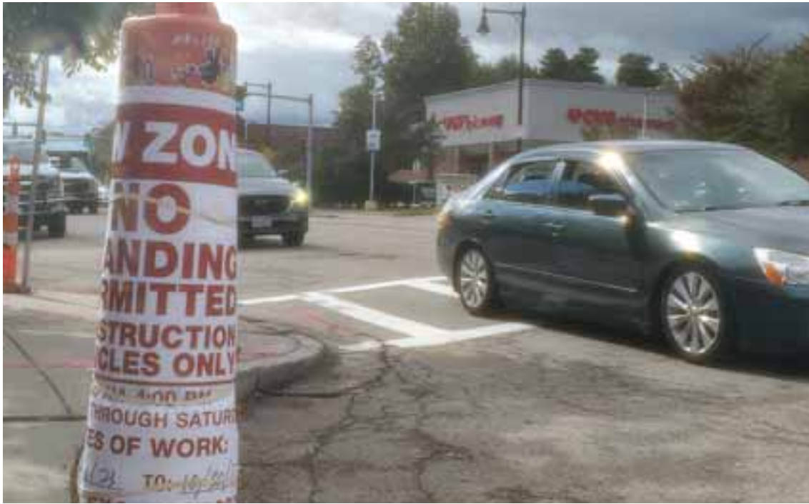
Road work has started on Centre Street in West Roxbury for the safety redesign and lane reduction of the street.
