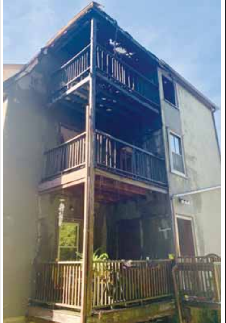
The Boston Fire Department responded to a call for a fire at a three-family home at 1932 Hyde Park Avenue. The Fire was reported around 3:30 p.m. on Sept. 22, and firefighters believe it was started on the second floor porches and extended to the third floor porch and the roof. No injuries were reported, but eight residents have been displaced according to the Red Cross and the chief on scene estimated the damage to the property at $250,000. Investigators have not yet reported a cause to have been determined for the fire.
