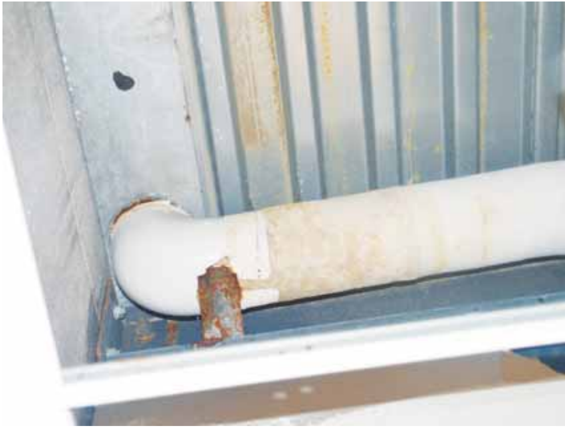
According to officials, the flooding appears to be coming from this pipe.
