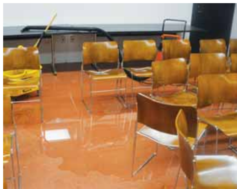
While there was no reported damage to books, the leaks in the library are growing and residents are worried.
