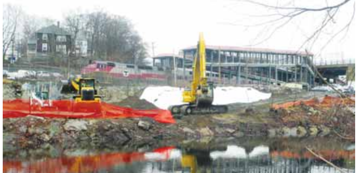
Crews are currently working on the former location of Lewis Chemical just on the banks of the mighty Neponset River in Hyde Park.
